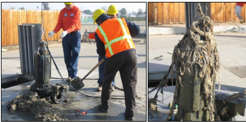
Wastewater treatment operators work on a pump clogged with wipes and other debris. (Photo provided by IWSFG)
